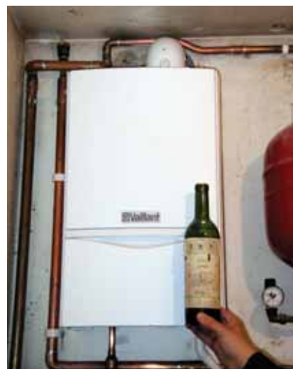
A condensing type boiler with bottle to show scale
